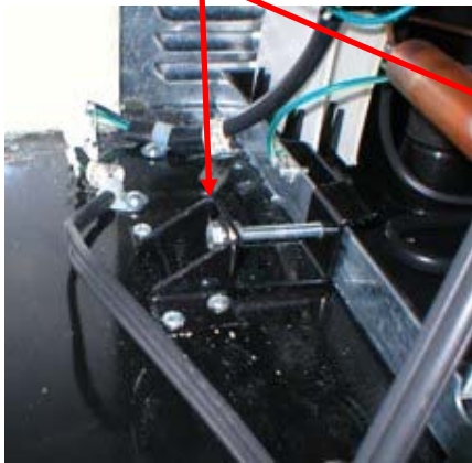
Refrigeration tie down bolt.
